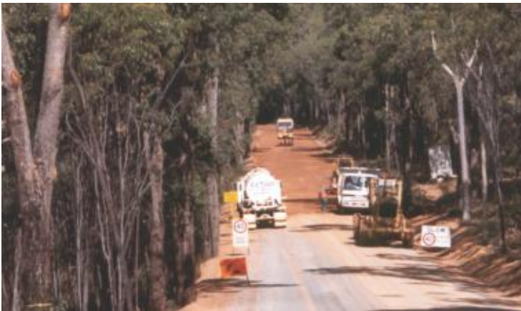
Road construction with Phytophthora Dieback infected soil or gravel can lead to the introduction of the disease into adjacent bushland.
