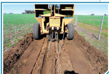
Chatfield Tree Planter available from Gillamii Centre drops seed on soil surface. Heavy chain aiming to cover coarse seed and fine chain to cover fine seed.
